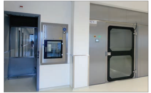
Image – Second level logistics barrier
