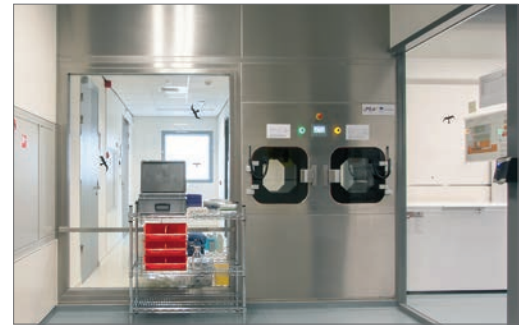
Image – First level small disinfection chambers
