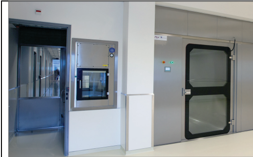
Image – Second level logistics barrier
