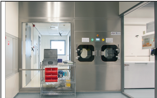
Image – First level small disinfection chambers
