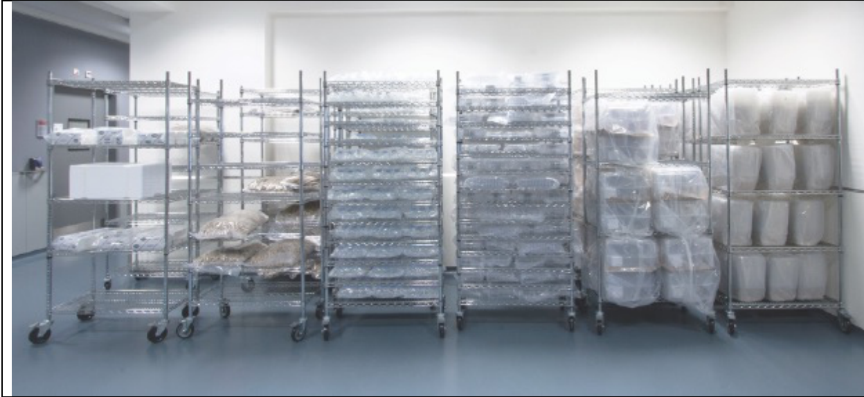
Image - Storage room for single-use cages and components
